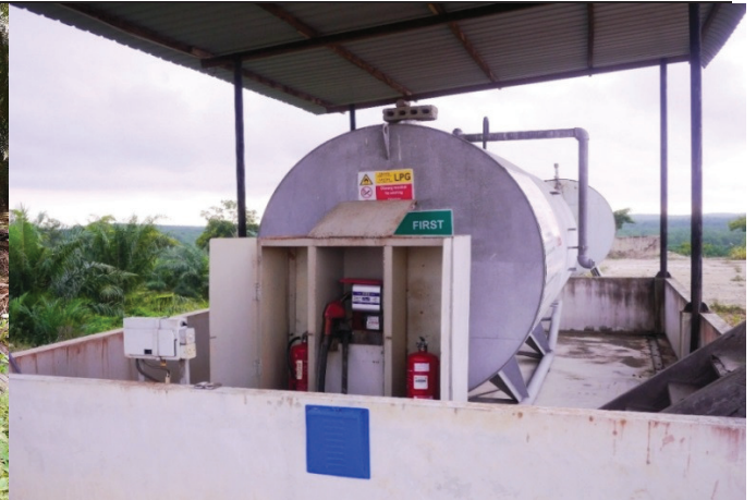
Lim & Lim estate: Secondary containment for Diesel tank
