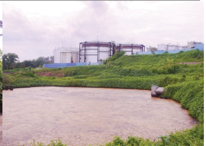
Masai POM: Newly commissioned Bio-Reactor plant
