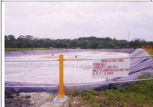
Masai POM: Newly commissioned Bio-Reactor plant
